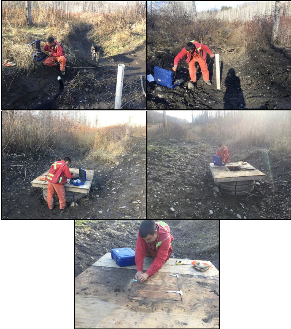
Figure 6: Photo Series showing examples of test and refuge pipe monitoring for groundwater level, temperature and DO in the fall of 2016 (October 31).
