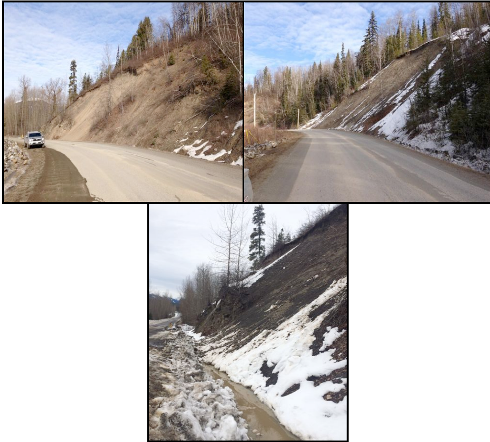
Figure 9: Failing hillslopes and turbid water flowing through ditch into the Kitwanga River looking north along the Gitanyow South Access Road (Photos taken February 2015).
